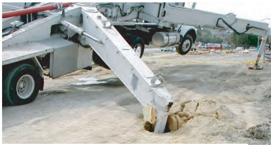
Figure 14 Hidden voids cause accidents
